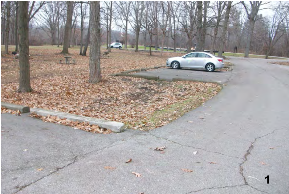
Existing parking lot to be restriped. Park entrance and toll booth in the distance.
