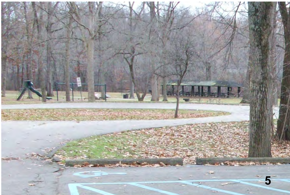
Catch basin in middle of circle to be removed, pipe abandoned in place. Circular turf area to be used as small retention area.
