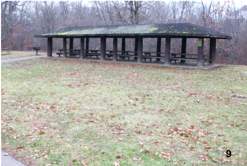
New universal accessible concrete access routes to be provided on both sides of the shelter. The existing walk exceeds 5%.
